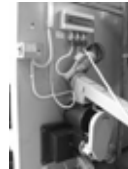
Burner charging feeder drive
